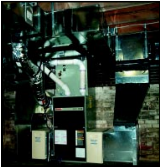
Photo 1 —Zoning an HVAC system requires more duct. Note that the gas exhaust goes through regular PVC pipe because it is cool. All of the furnace controls are located in the lower cabinet.
