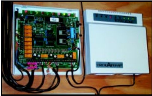
Photo 4 —These zone panels handle three thermostats. The thermostats and dampers are wired at the bottom, and the HVAC system control is wired on the left. Numerous indicators show the system's status, including the state of each damper. Monitoring panels with an HA system with buffers is easy.
