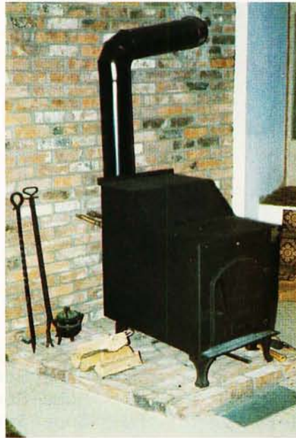
Photo 1: The Hydrostove is installed in the corner of the Circuit Cellar. Take note of the two copper pipes coming out the rear of the stove into the wall. The pipes, which are buried behind the wall and above the ceiling, go to the furnace, which is 35 feet away.
