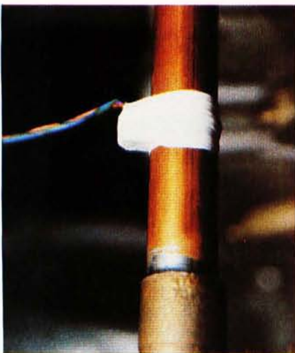
Photo 6: To effectively use this control device, it is important to have accurate temperature measurements. The LM334 temperature sensor is easily attached to the Hydrostove return pipe by wrapping Teflon plumbing tape around it.
